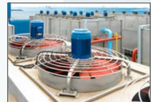
Fans and water pumps
